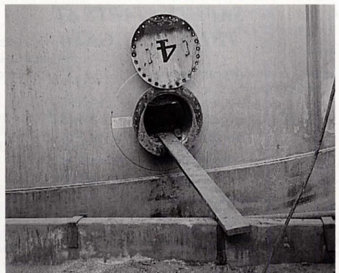
Potential hazard - cover not secured (or removed), and inadequate means of access.
