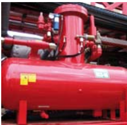
Air-oil separator tank
