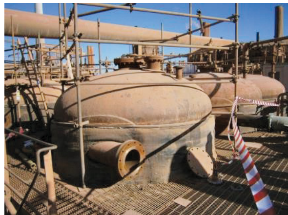
Top level of the digester bank showing disconnected pipework
