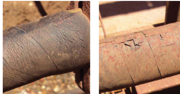
Flexible rubber hoses showing external damage. Only testing by a competent person will reveal whether the internal integrity of the hose has been compromised
