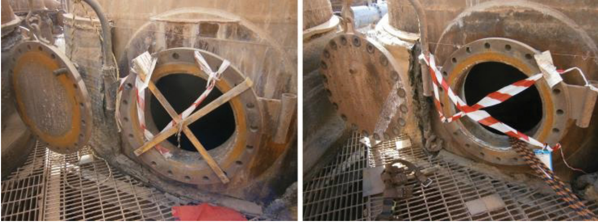
Left: Manway into a digester with mechanical guard fitted. Right: Manway entry for the digester without scaffolding (tape placed by emergency response team)
