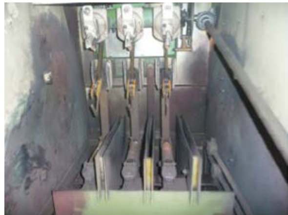
Figure 1 Photograph of the switchgear cabinet showing damage from the arc blast
