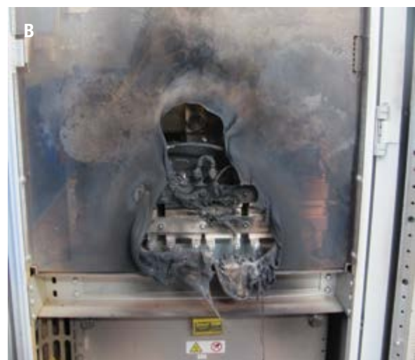
Photographs showing (A) location of initial short circuit fault in the VSD and (B) resultant arc damage to internal components
