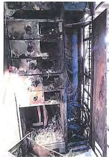
Damaged MCC modules
