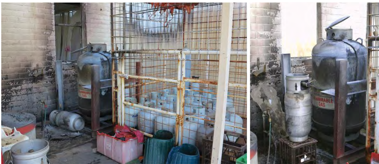
Left: Safety shut-off valves forming part of the burner management system. Right: Damage to boiler
