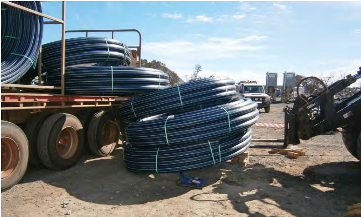
Position of poly pipe after the incident. The forklift and hydraulic jacks were used to move the poly pipe to access the underground operator trapped beneath.
