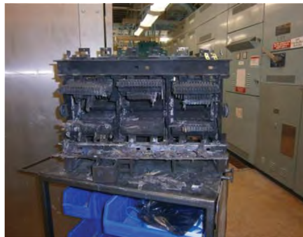
Damage to 4,000 A switch following incident
