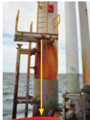
Photographs showing location of handrail attachments that failed (top) and fall path from landing (bottom)
