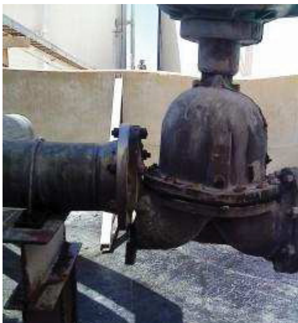
Valve damaged during third acid spill
