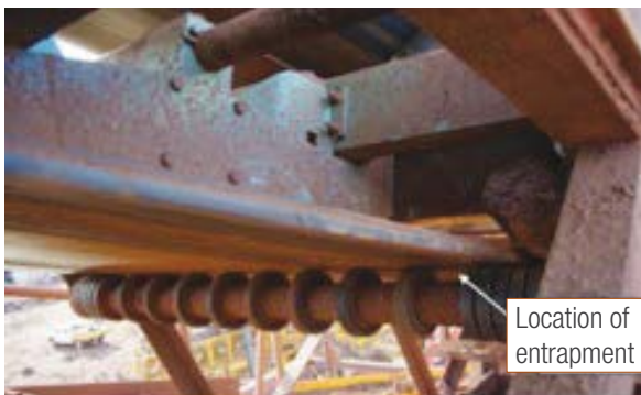
Photographs showing calibration weight requiring cleaning (top) and nearby return roller (bottom)
