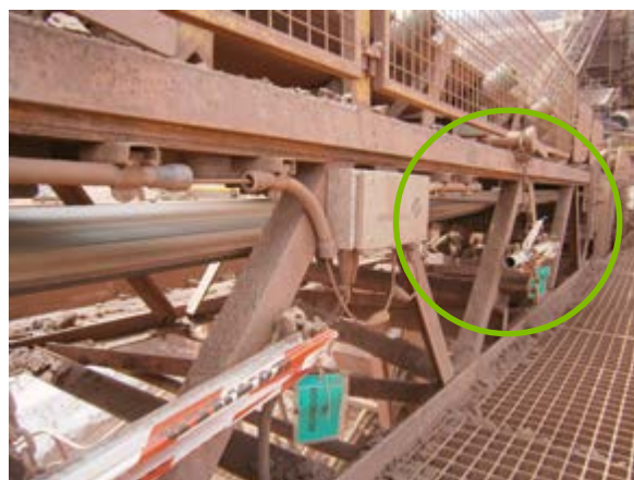
Photographs showing location of weightometer under conveyor belt
